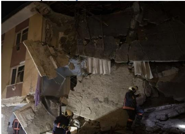
b) Structural damage due to an explosion happened on an apartment building in Ankara (NTV, 2022)
